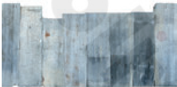
Fig 10.7 Damaged iron sheets
