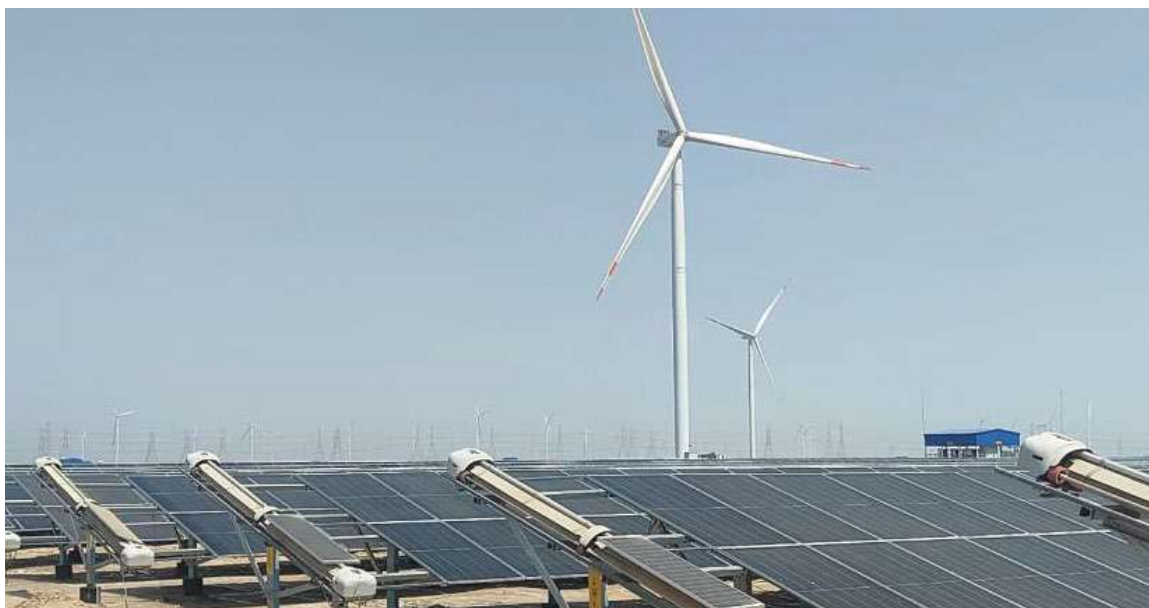
1,363 MW hybrid renewable energy greenfield project (solar and wind) in Khavda, Kutch district, Gujarat, supported under NGLF
