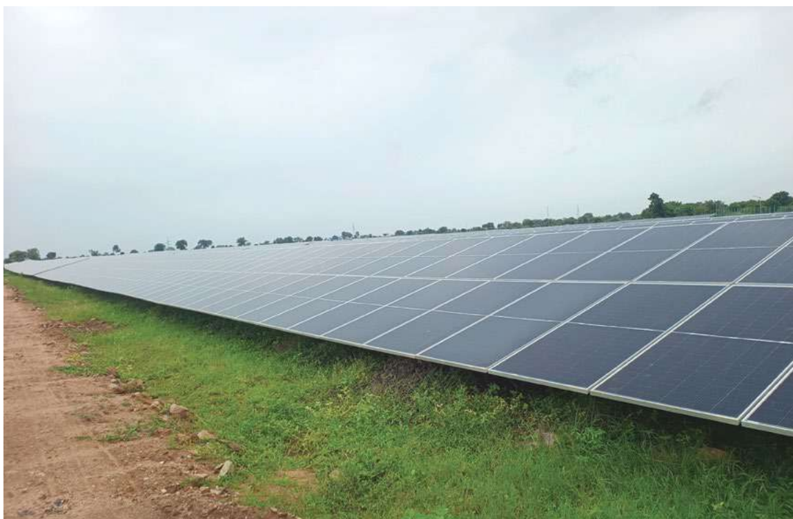
70 MW (AC)/97 MW (DC) solar photovoltaic project at Hongunta village, Kalaburagi district, Karnataka, supported under NGLF
